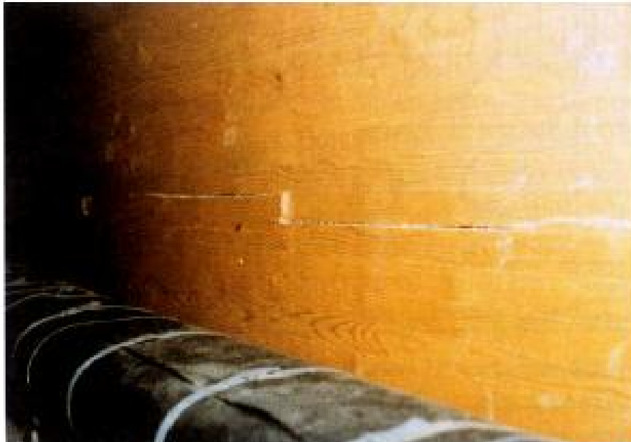
Fig. 9. Longitudinal through crack in glulam roof girder due to shrinkage effects. Hot water piping in the vicinity of the girder contributed to fast drying. Source: Ref. [7].
