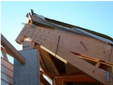
Figure 2. The corner has concealed steel plates which connects the timber parts. Between the visible bolts numerous dowels are placed.
