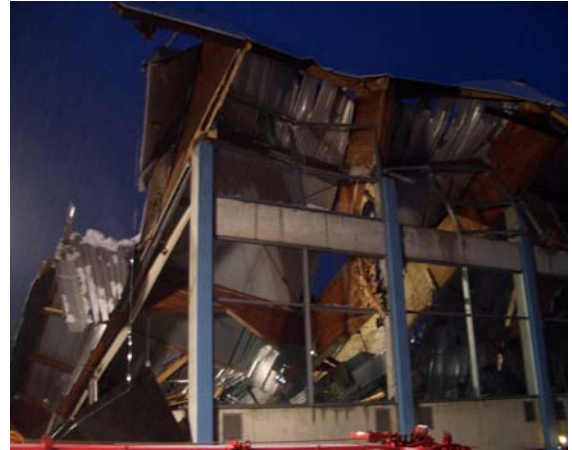
Figure 2: Partial view of the collapsed roof structure
