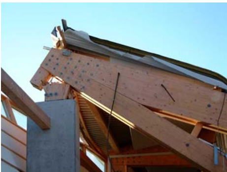
Figure 2. The corner where concealed steel plates connects the timber parts. Between the visible bolts numerous dowels are placed.
