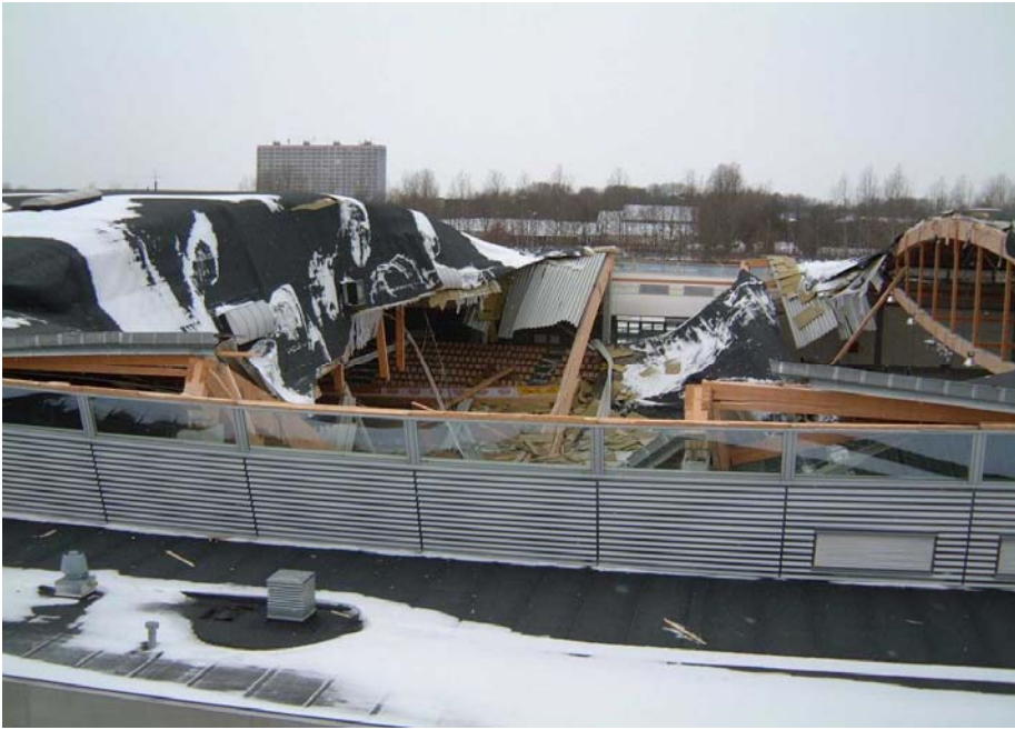
Figure 1. The roof of Siemens Arena after the collapse of two trusses. An intact truss is seen to the right.
