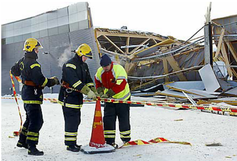
2500 m 2 of roof fell down: Typically high consequence
