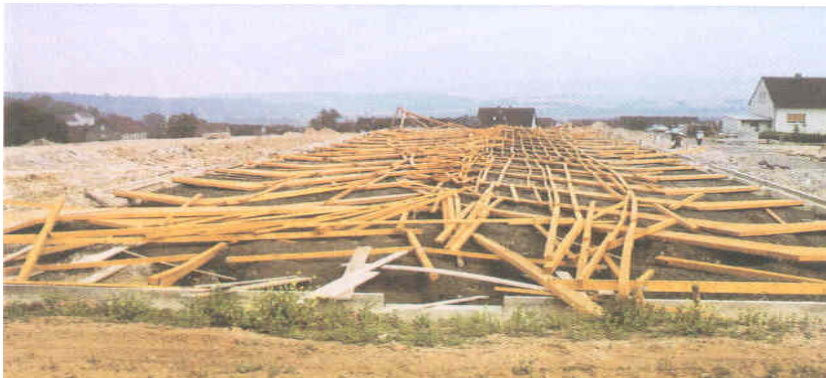
Collapse (one of the 79 cases)
