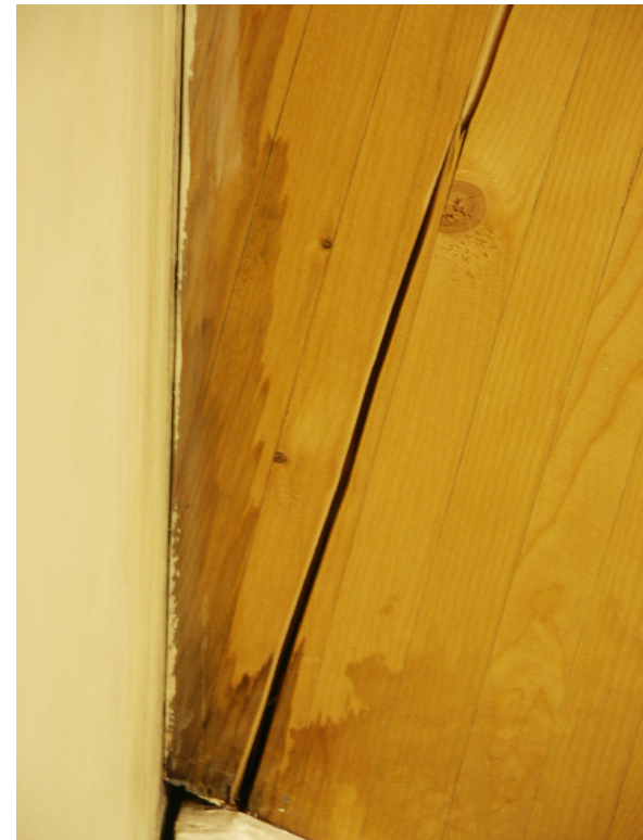
Crack in glulam arch Typically low consequence
