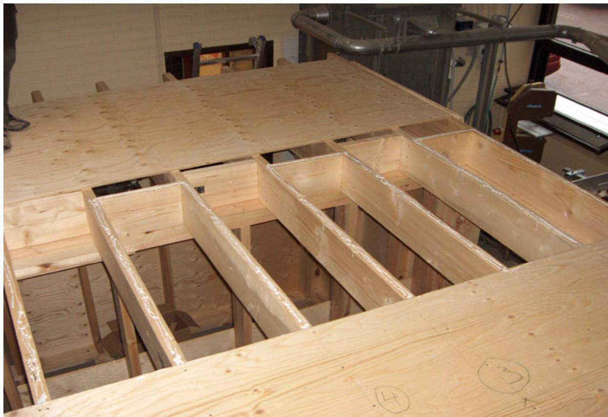
Figure 1: Typical Finnish floor, similar to the test floor described: constructed with main solid timber beams, blocking elements, tension bar and plywood deck
