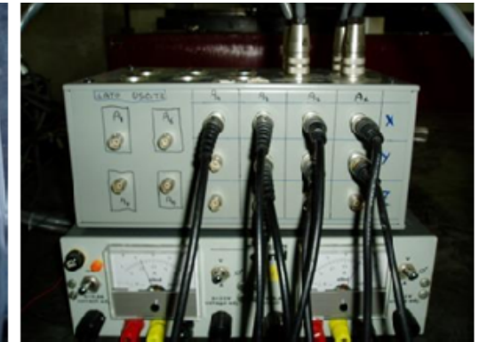
b) Junction box lateral view: 8 outputs to the acquisition
