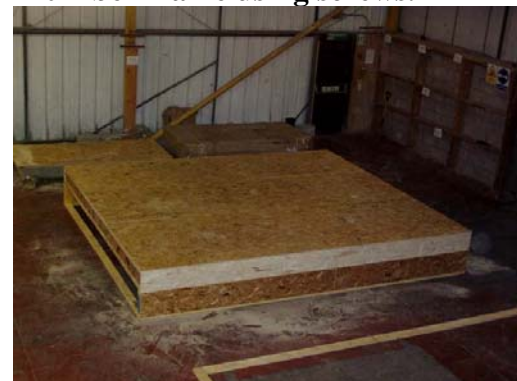
(d) The floor, decked with OSB and supported in two edges, was finished.
