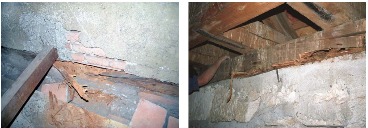
Figures 15, 16: Destroyed supporting beams of roof structures
