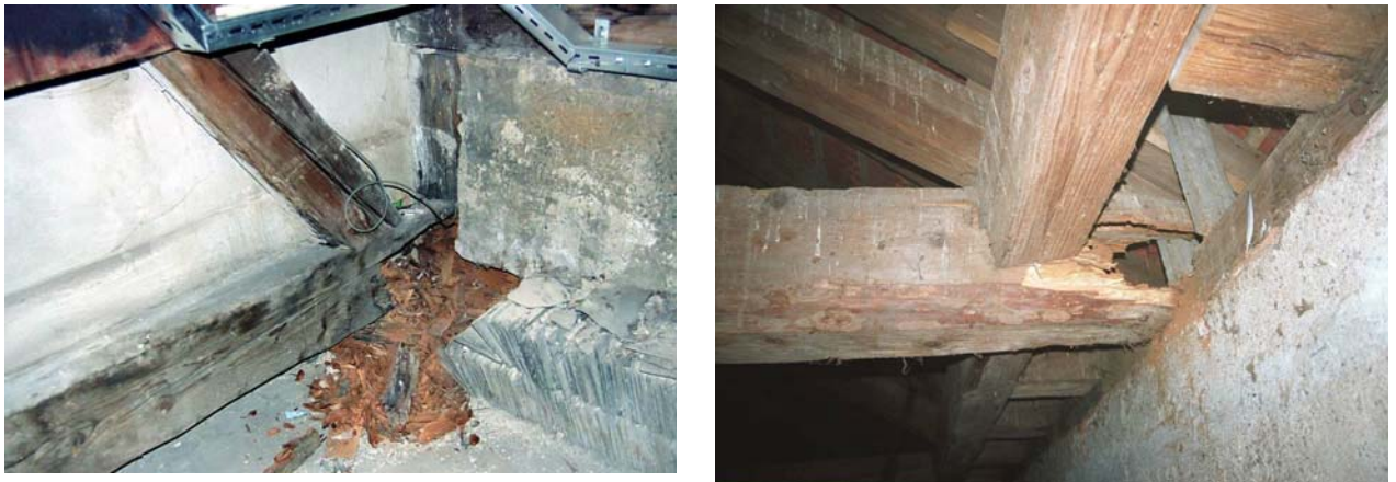
Figures 13, 14: Failed lower chords of roof beams
